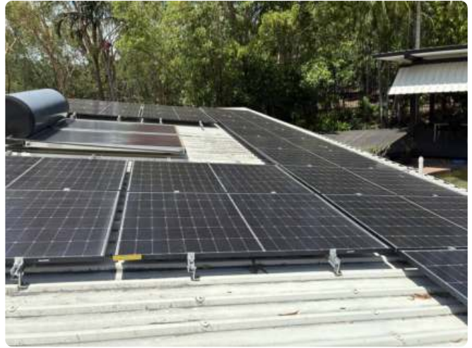
590-4080-9 Pv Solar System
