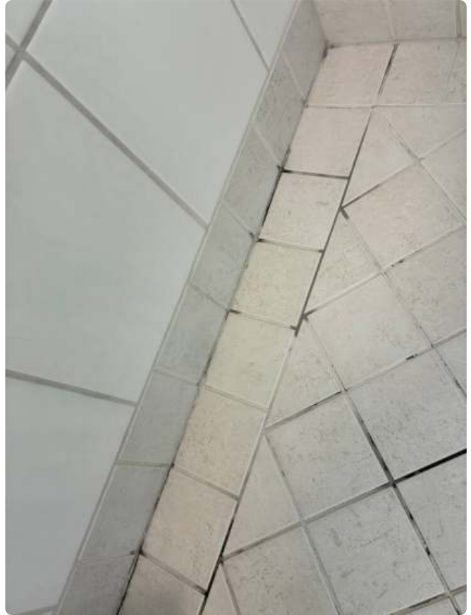
Significant defect to flooring tiles on the surface of shower area.
