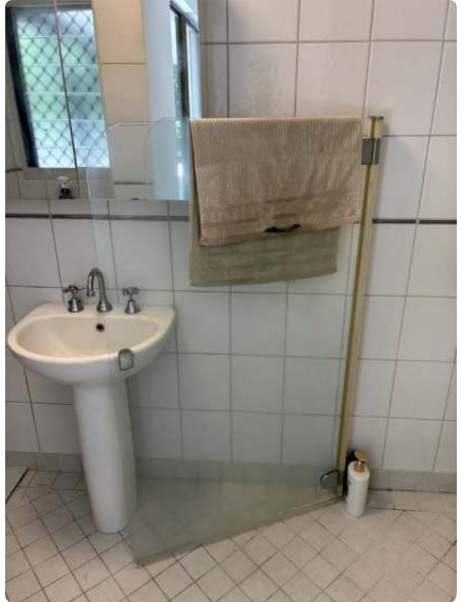
Screen door is stiff and heavy to open.
