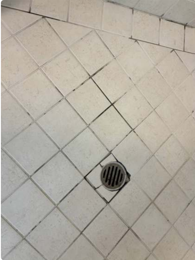
Significant defect to flooring tiles on the surface of shower area.
