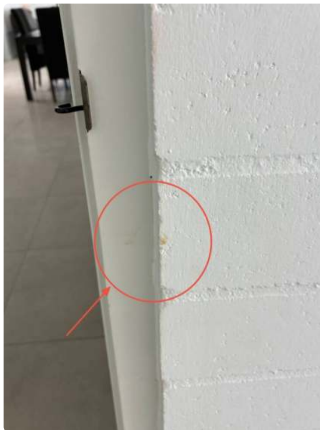
Minor staining on wall and door frame.
